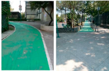
Figure 4. Bicycle tire brands due to excessive speed in sharp turns and lack of confined lane
